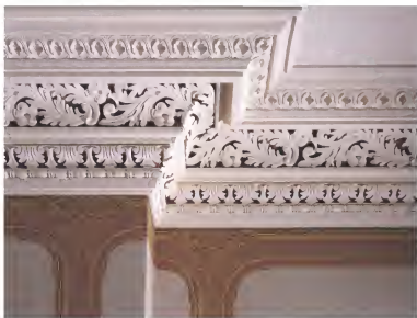
Detail of the intricate cast plaster cornice that runs around the perimeter of the room. After precise molds were made from samples of the original plasterwork, a new cornice was cast for the room's installation.
